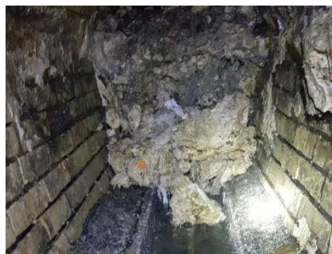
Figure 1: A 10 tonne fatberg discovered in a London sewer in 2020 (BBC, 2020)
